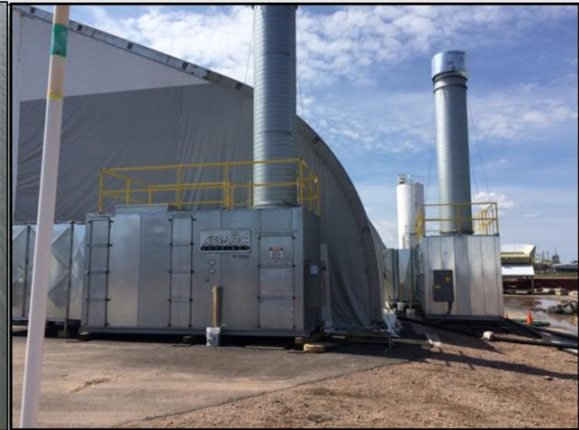
Vapor Phase Odor Control System
