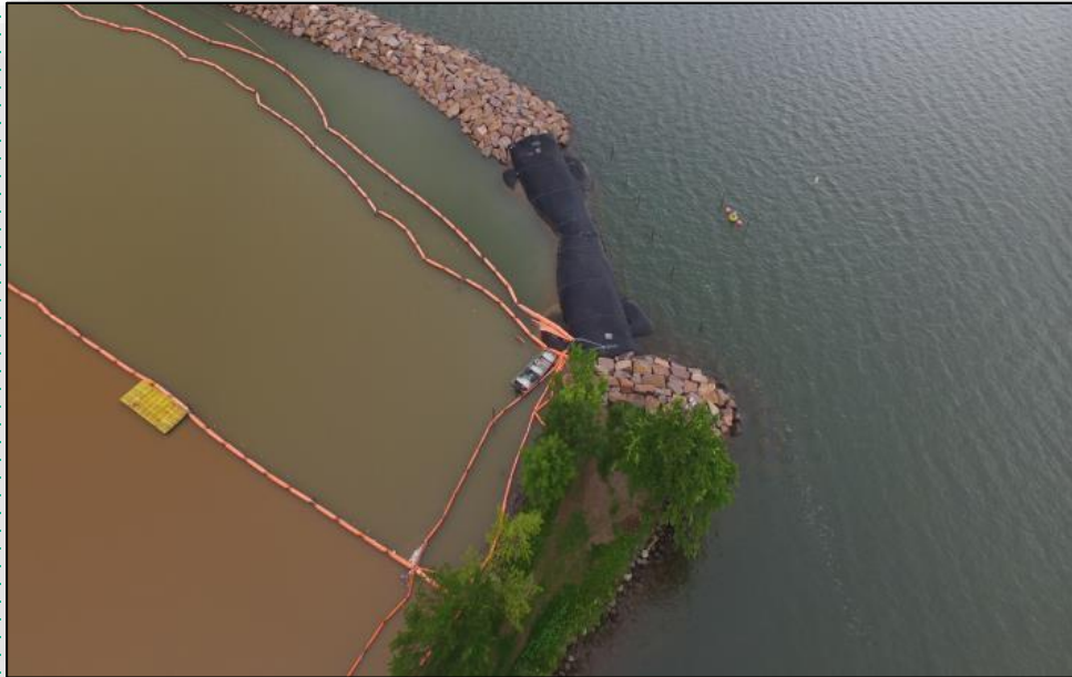
Multiple Barrier Curtain System to contain work area impacts and protect Lake Superior
